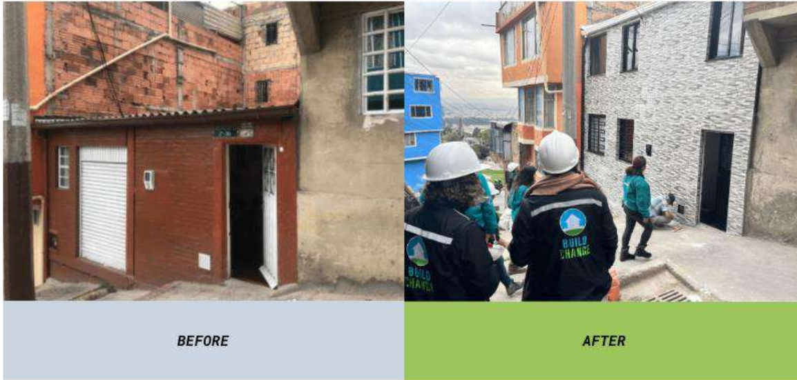
Ercilia Suarez's house before and after retrofit and vertical expansion under the city of Bogotá's Plan Terrazas program, supported by technical assistance from Build Change.
