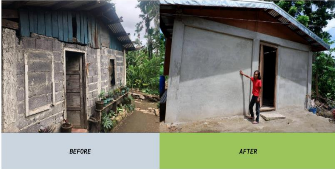
Before and after: Homeowner Josefina Hagosojos's house was part of a home improvement intervention in The Philippines
