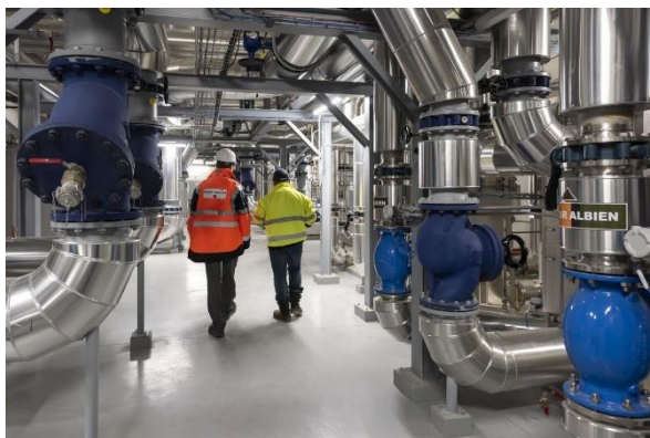
The 5th generation heating and cooling grid of Paris-Saclay in France - ©Carlos Ayesta, EPA Paris-Saclay
